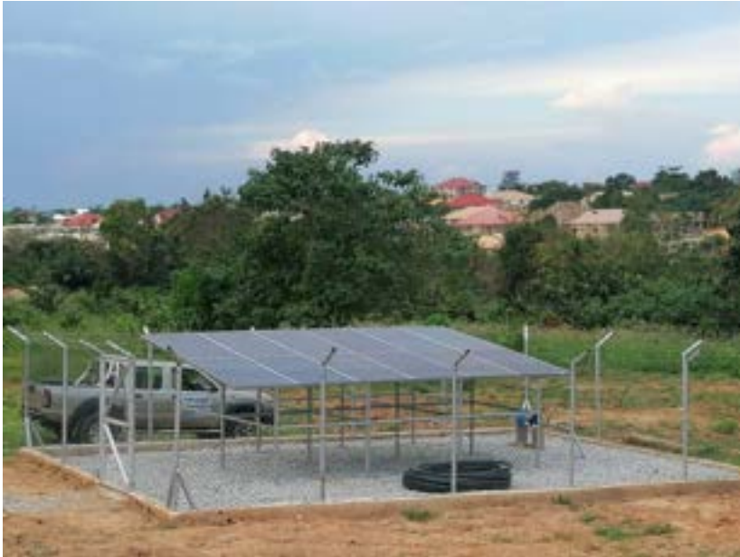
3960watt array at a farm
